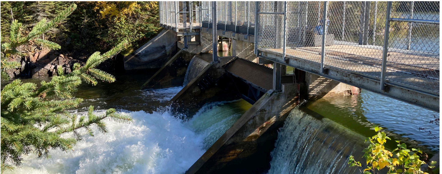
Environmental - Rapid River Dam submitted by Trenton Spence, PTech
